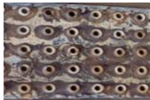
Fig. 3. Exchanger mirror with the presence of corrosion and incrustations
